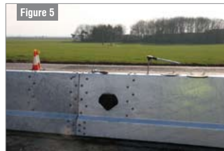
Access hatch in DSSB unit
