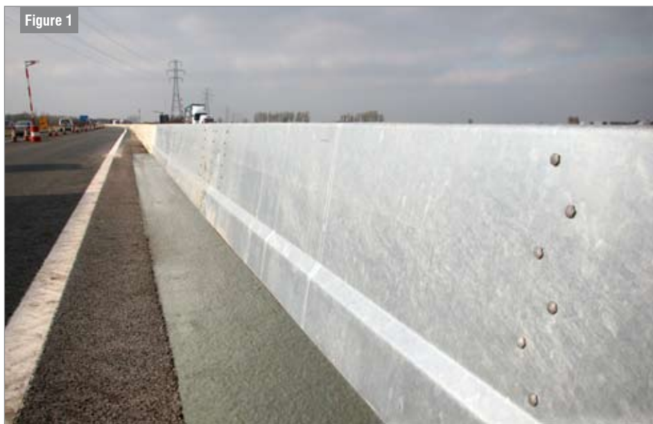
Figure 1 Typical ECP installation
